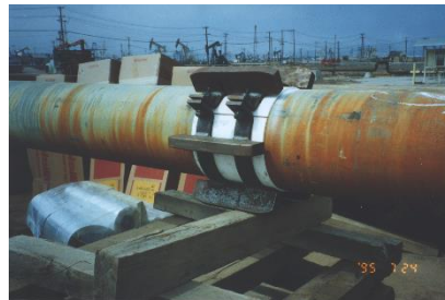
RS-101 Cylinder were used an eutectic insulator to prevent corrosion in a underwater oil pipeline.
